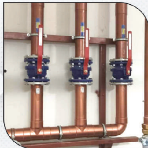
MEDICAL GAS PIPELINE SYSTEM
